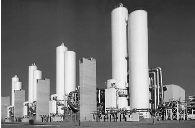
Fig. 1.3 Air separation unit at Cantarell, Mexico (2000).
